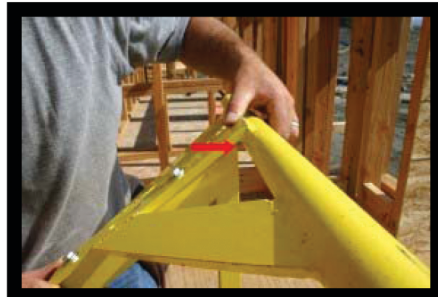
3. Before tightening bolts, make sure cross member has a gap between mainframe and flat weld on cross member.
